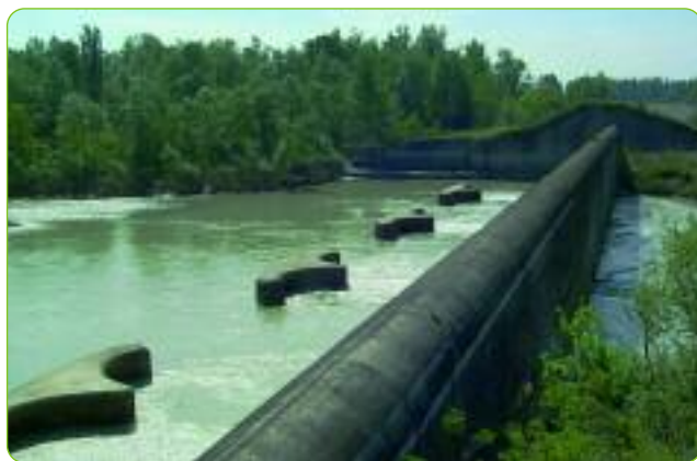
Water infrastructure at the Secchia River Nature Park. Photo by Claudio Chiossi
